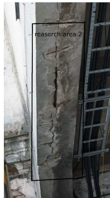
Figure 3. The research object 2- concrete element with the cracks
