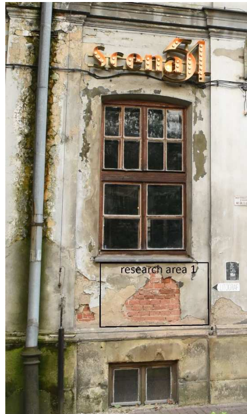
Figure 2. The research object 1- wall with damaged plaster
