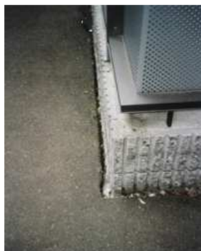
Gap generated between block and pavement
