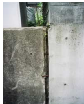
Crack running in concrete retaining wall
