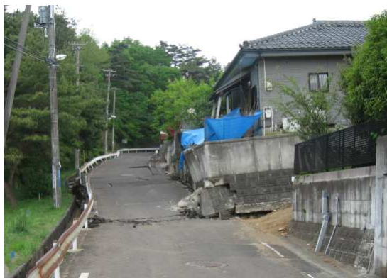
Landslide in Oritate Area Building sliding over the road, which used to be straight is curving now
