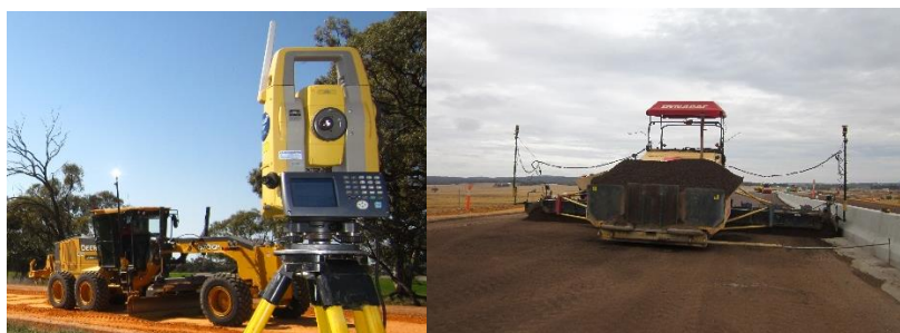
Figure 2. (a) Motor-grader using automatic blade control with Robotic Total Station for fine grading. (b) Tracked Paver controlled by GNSS and Millimeter GPS laser system. (Position Partners 2015)
