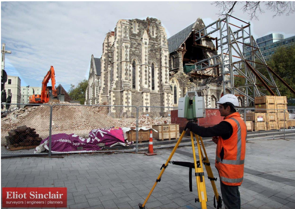
Figure 4 - Christ Church Cathedral (Rose Window Collapsed)
