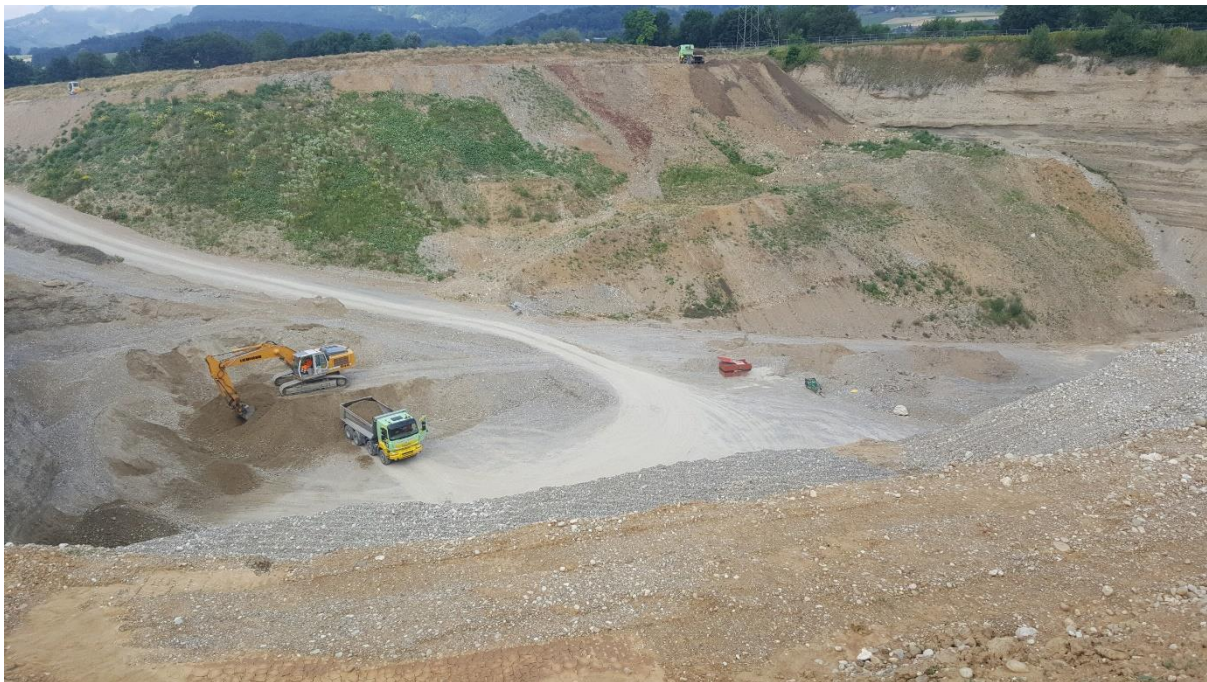
Figure 1: The project site, a four–hectare gravel pit in Lostorf near Olten, Switzerland
