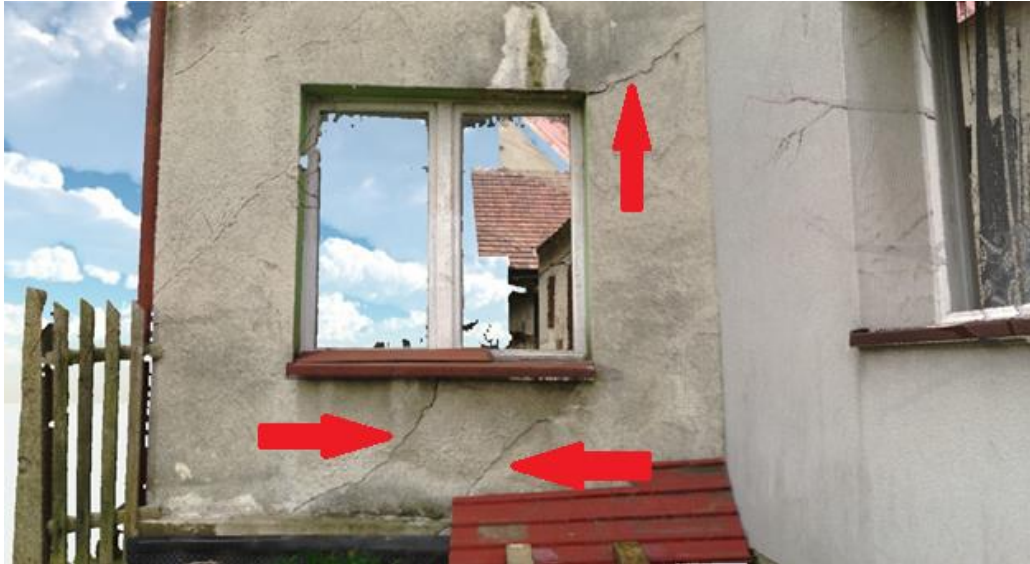
Fig. 8. Cracks in the building wall - model created on the basis of data from a stationary scanner (source: own study)
