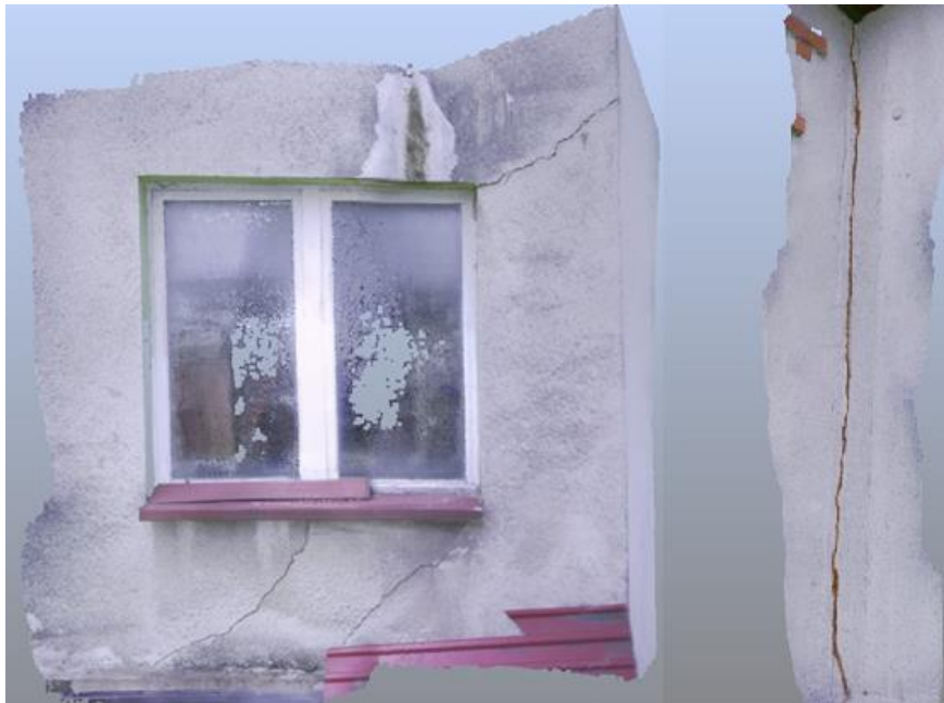
Fig. 9. Cracks in the walls of the building - models created on the basis of data from a handheld scanner (source: own study)
