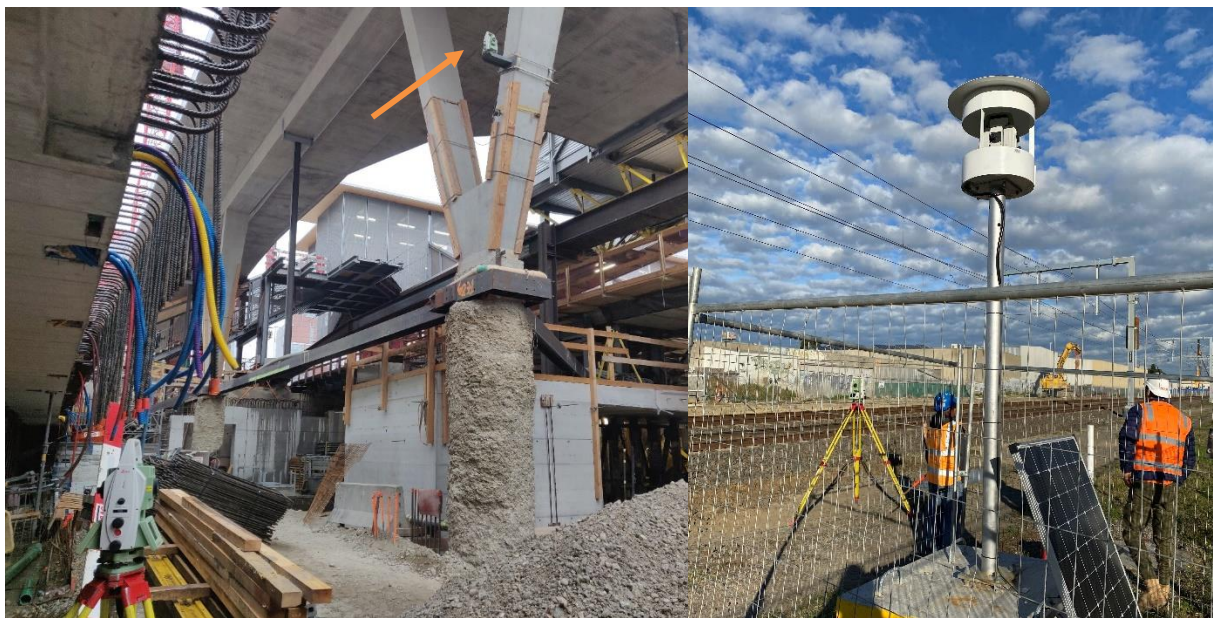
Figure 10 Surveying and monitoring of a railway platform construction in Switzerland and Australia
