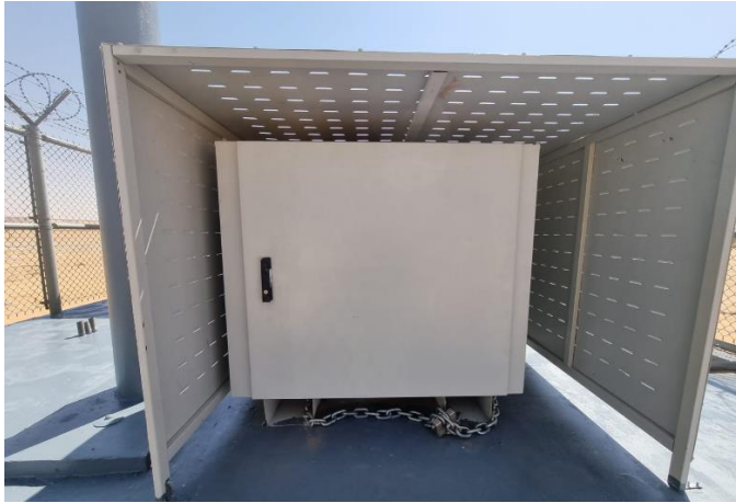
Figure 6: KSA-CORS Cabinet protective layer
