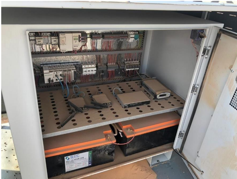
Figure 2: : KSA-CORS IP66 Internal Cabinet filled with Dust
