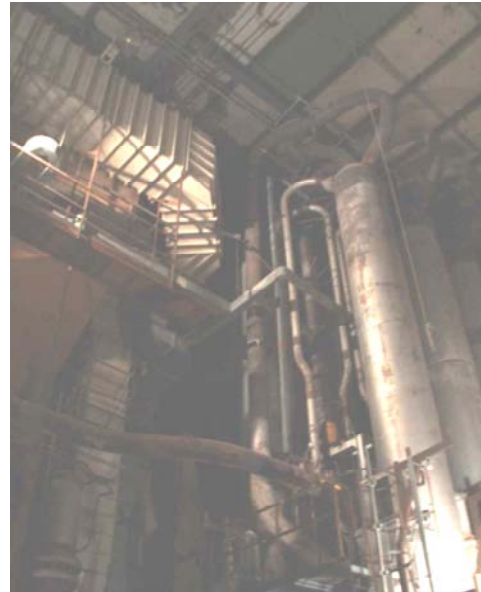
Exchanger in situ
